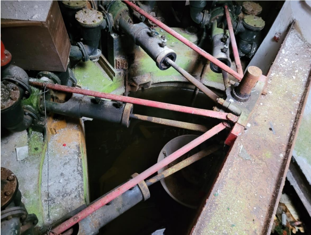
Figure 1.4.7 Turbines in the Old Waterworks (photograph taken by Arup on site visit)
