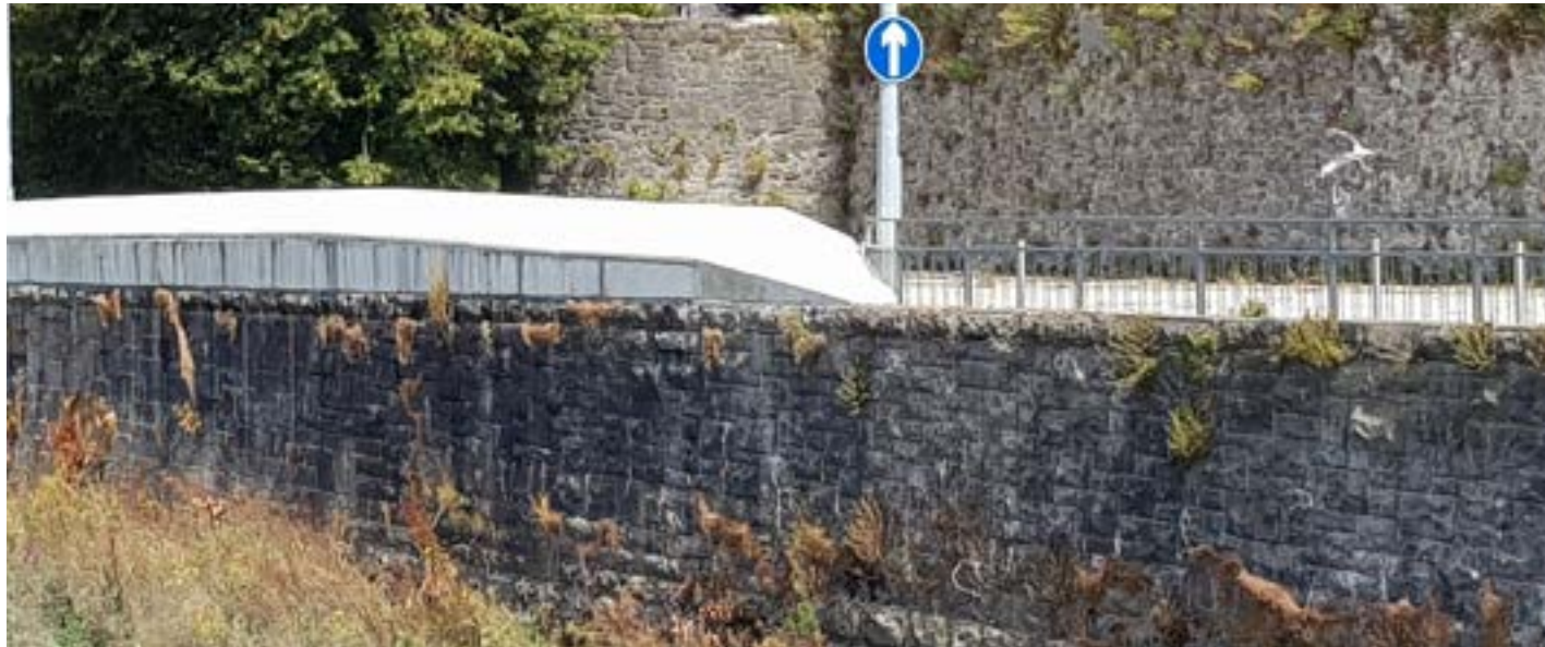
Riverside view of the upgraded wall and connection with the existing wall and railing.
