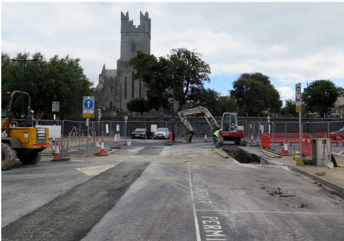
Figure 92 Northeast-facing view of St Mary's Cathedral with excavation of TT5-3 to right
