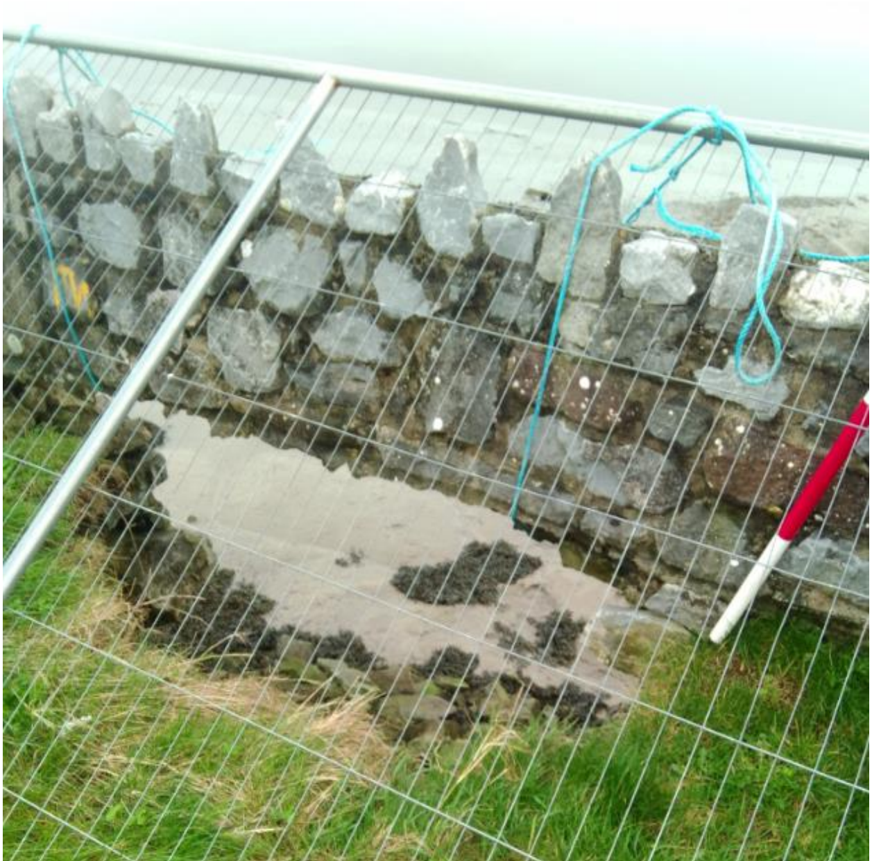
Figure 6.7: Survey Imagery Showing Damage to Blennerville Wall nearby XS250
