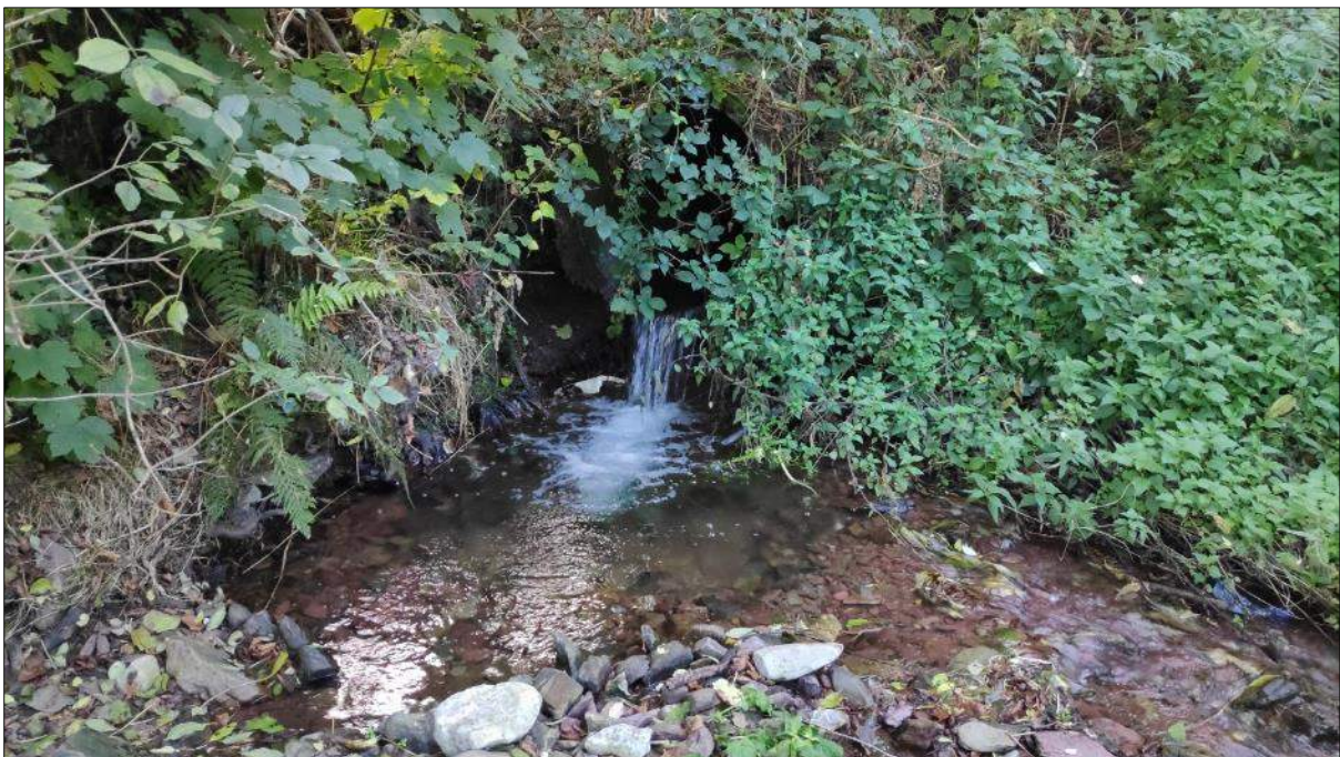
Plate 3.12 Confluence of the Lisnahorna Stream with the Glashaboy River via a perched pipe culvert (significant barrier to fish migration at base flows)
