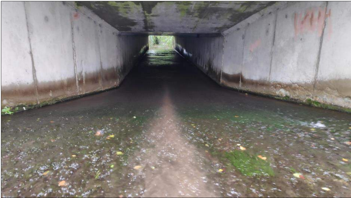
Plate 3.21 Sloping box culvert present at site 9 on the Lisheenroe Stream (a significant barrier to fish migration)
