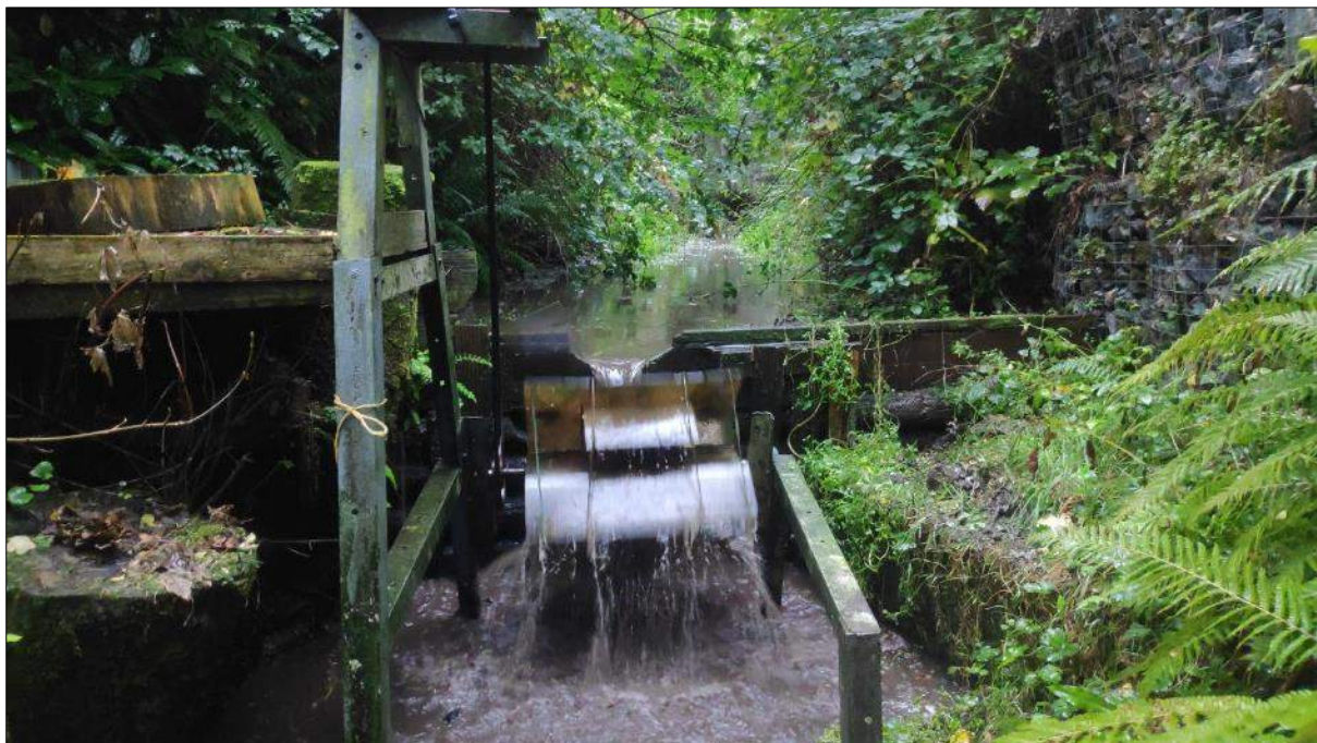
Plate 3.16 Representative image of site 7 on lower reaches of the Rathcooney Stream showing locally-installed hydro-electric turbine, September 2022 (significant barrier to fish migration)
