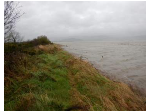
Figure 8 The Lord Limerick embankment photographed Jan-2020, with the sea completely submerging the marsh area. (See Figure 1 for a comparison to normal conditions).
