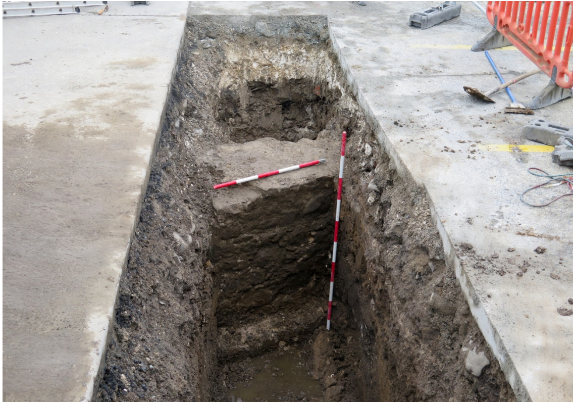
Figure 60: TT4-4, looking SW to rear of 1760's quay wall on plinth (compare to wall found in TT4-1).
