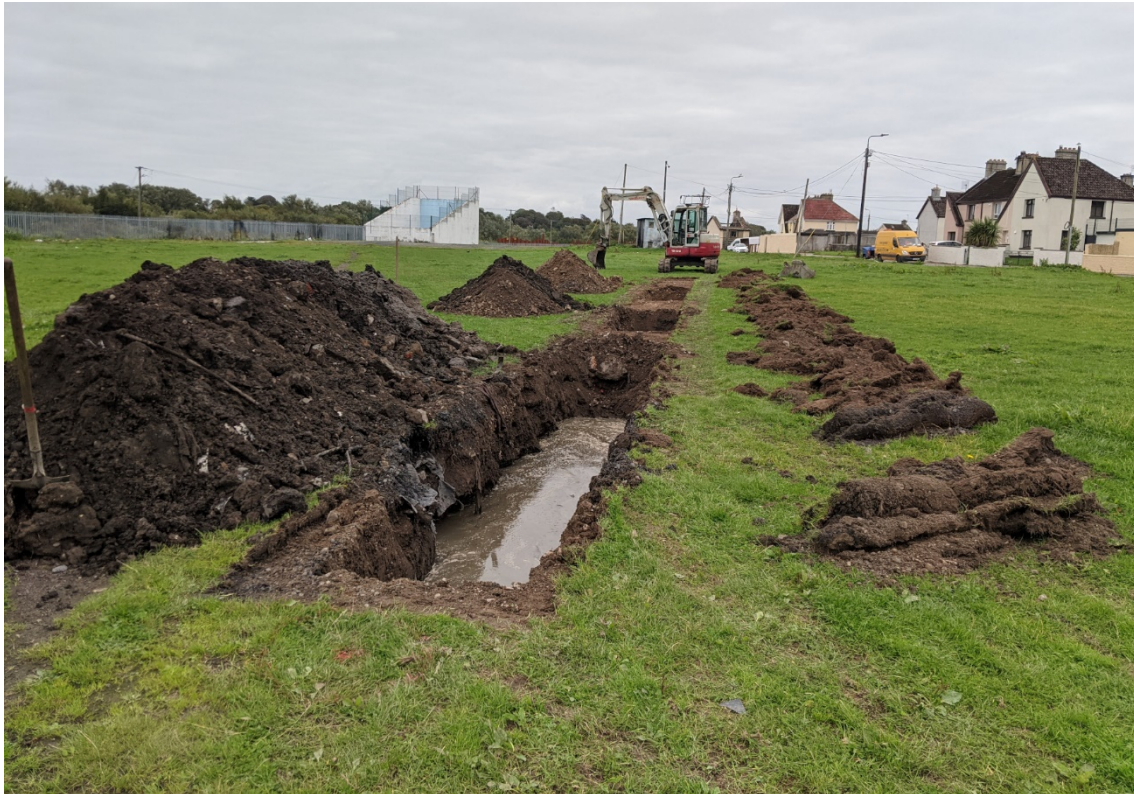
Figure 176 TT9-1, east-facing view. Note flooding from trapped water.
