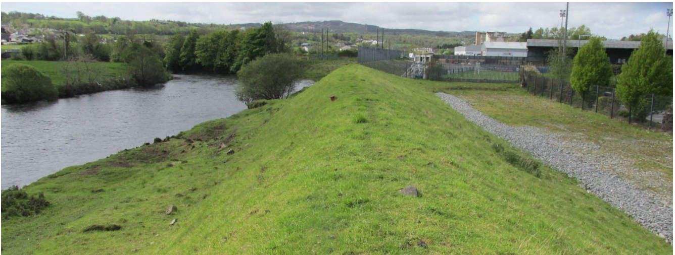
An image of the existing embankment at Ballybofey which will undergo further investigation work to determine its condition
