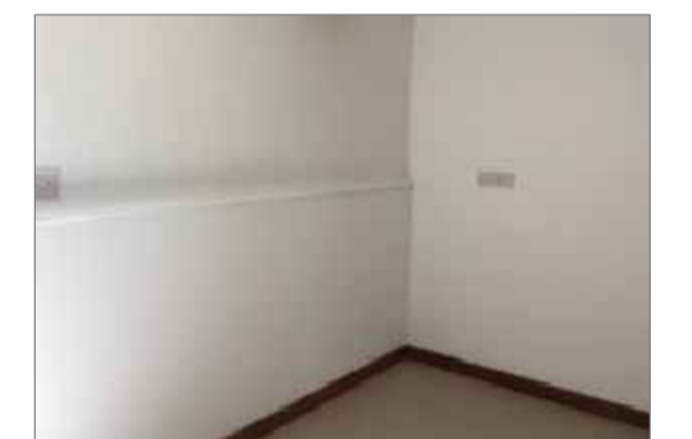
Raised Electrical Sockets
