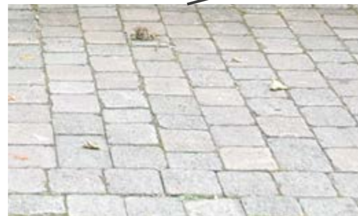
Existing sett paving and soldier course between Abbey Bridge and Baal's Bridge
