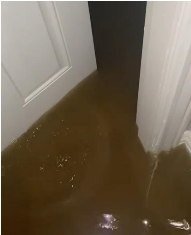
Figure 2-3 - Internal Flooding of The Maples Housing Estate (28 th October)
