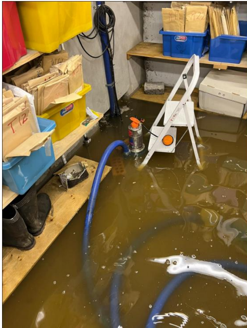
Figure 2-19 - Basement Flooding of GV Maloney & Co. Solicitors
