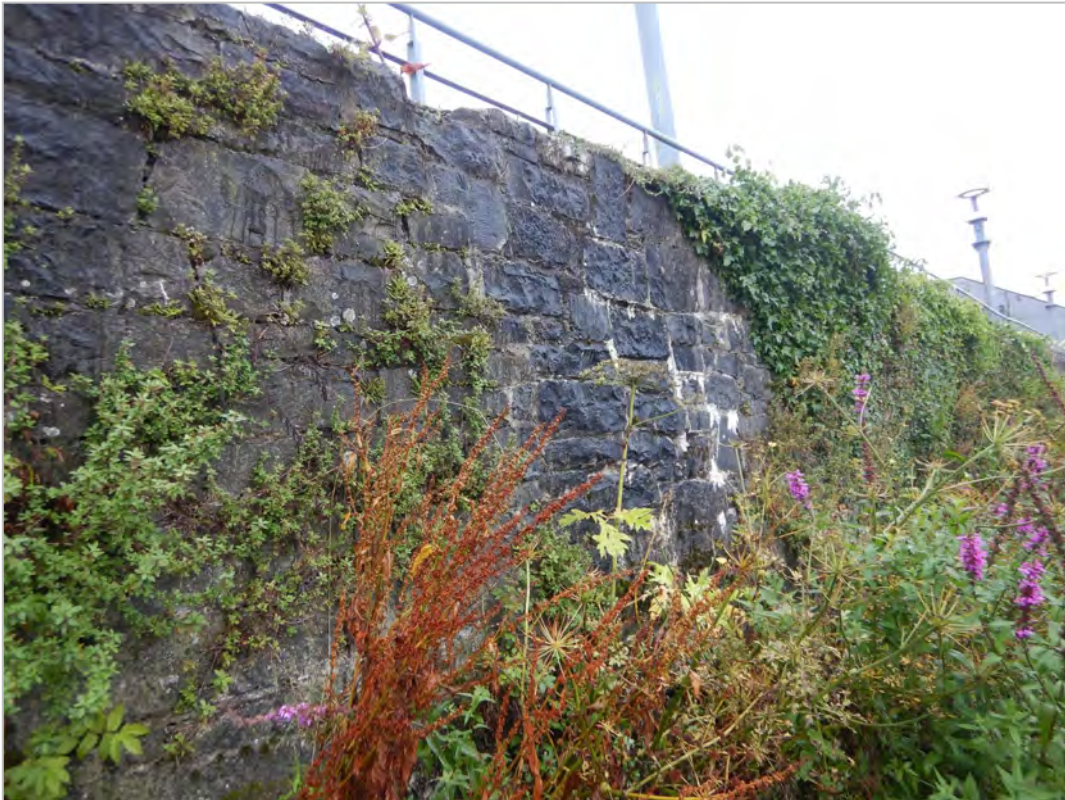
Plate 13 Quay wall immediately south of King John's Castle, highly vegetated and with evidence of repairs, taken from north west.
