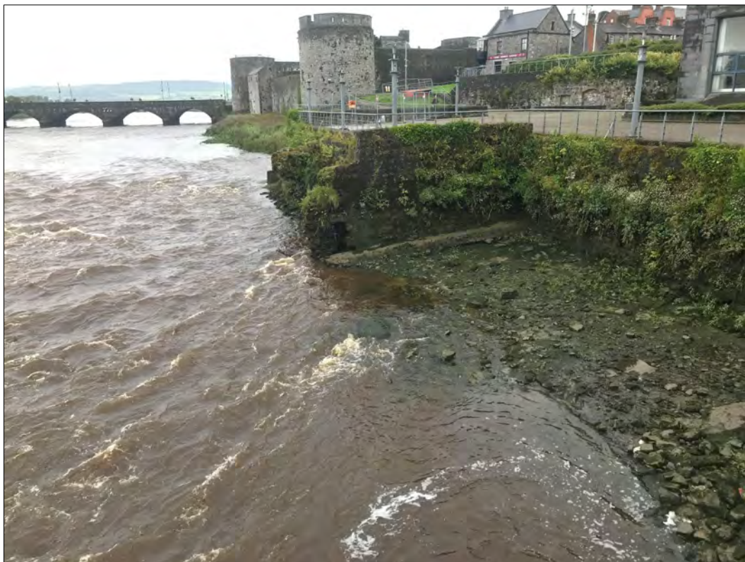
Plate 17 View north from 'inlet' showing wall remains in the mid ground with outfall pipe at base, taken from south.
