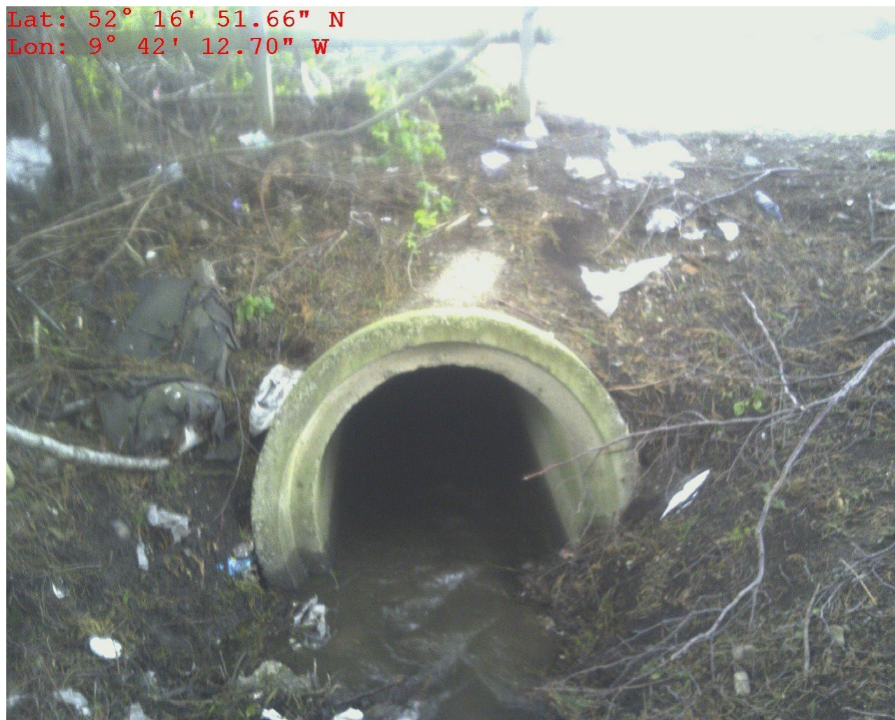
Figure 3.59: Inlet of Balloonagh Long Culvert
