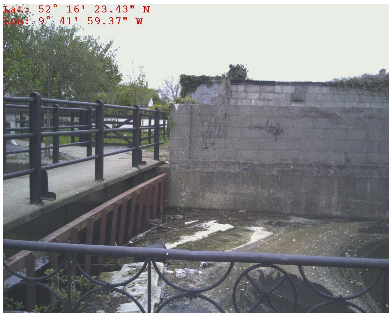
Figure 3.62: Debris caught in Trash Screen
