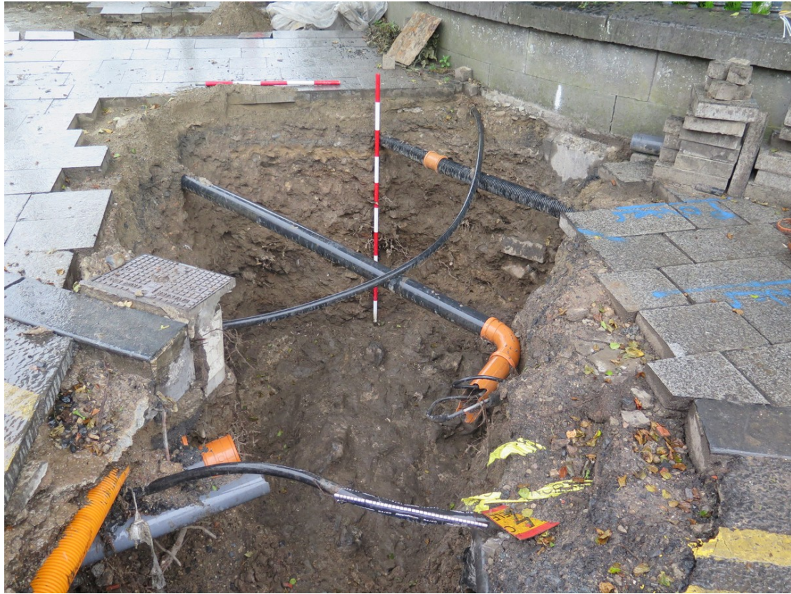
Figure 126 Looking towards corner of Potato Market showing Stone foundation of possible bastion
