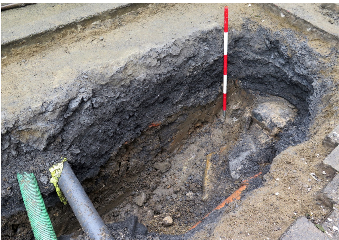
Figure 169 Southeast corner of TT7-4 showing services and collapsed culvert
