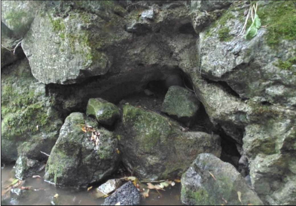
Plate 1.1 – Suspected Otter Holt (excavation under collapsed riverine retaining wall)
