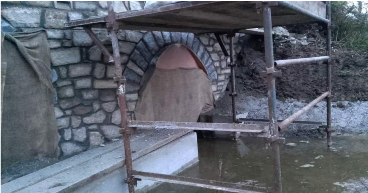
Photograph 2 Example of canvas sheets used to close off the bridge arches once they have been declared bat free by a Bat Specialist.
