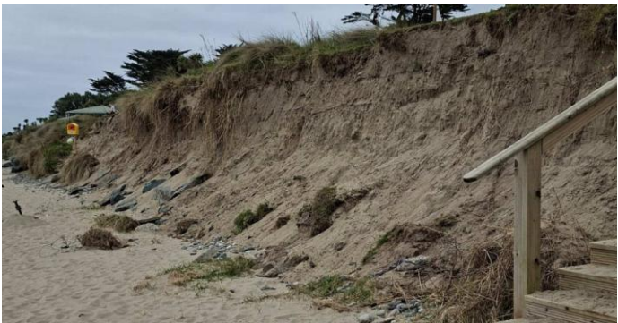
1: Erosion at Kellys Resort in January 2026
