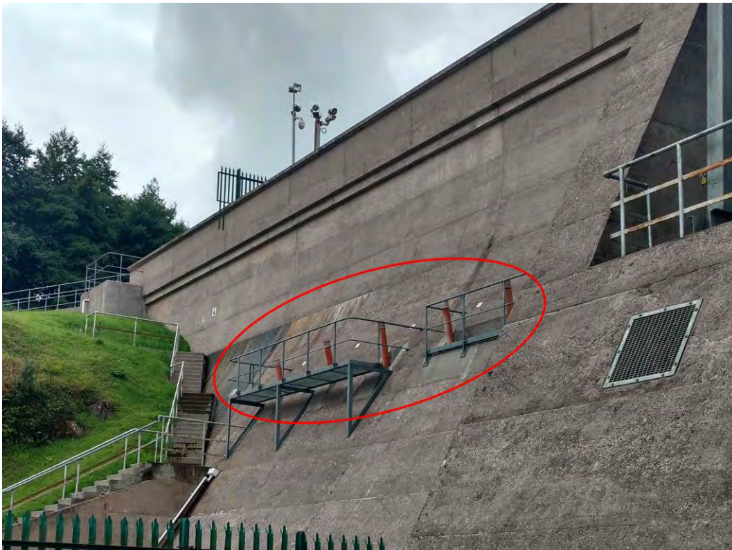
Figure 15: Downstream face of Carrigadrohid Dam, showing existing anchor heads in close proximity to each other
