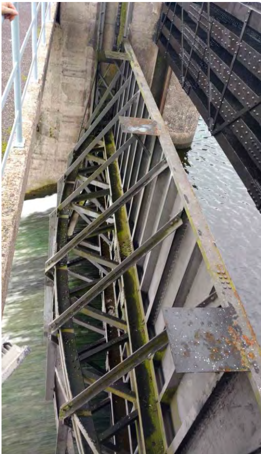
Figure 20: Typical Inniscarra Spillway Gate
