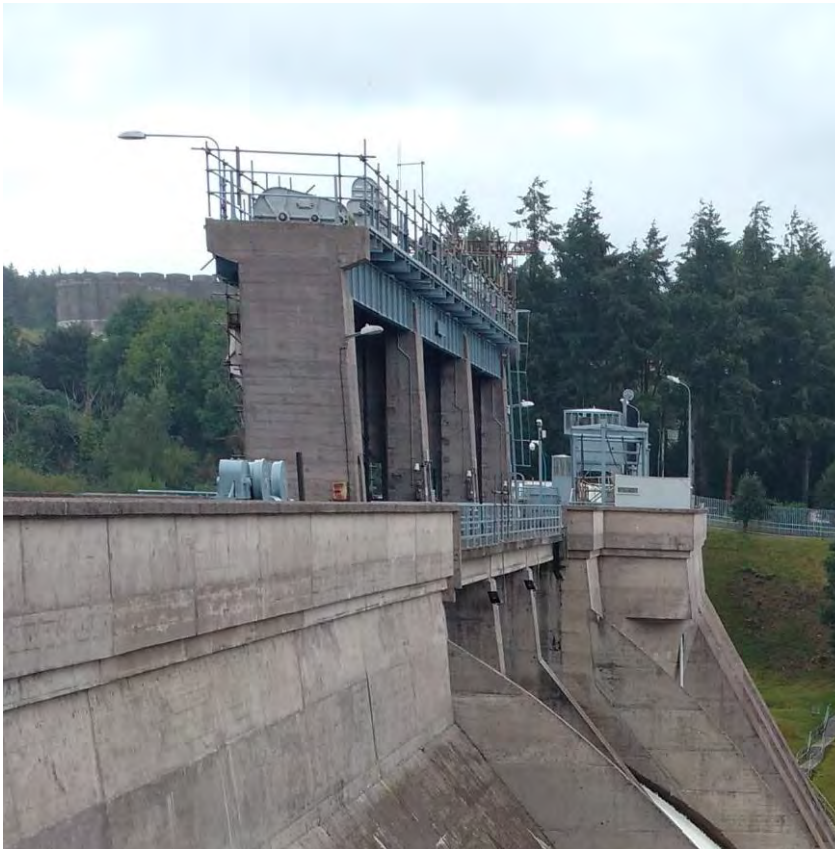
Figure 18: Inniscarra dam crest, showing sluice gate lifting gear and supporting concrete piers
