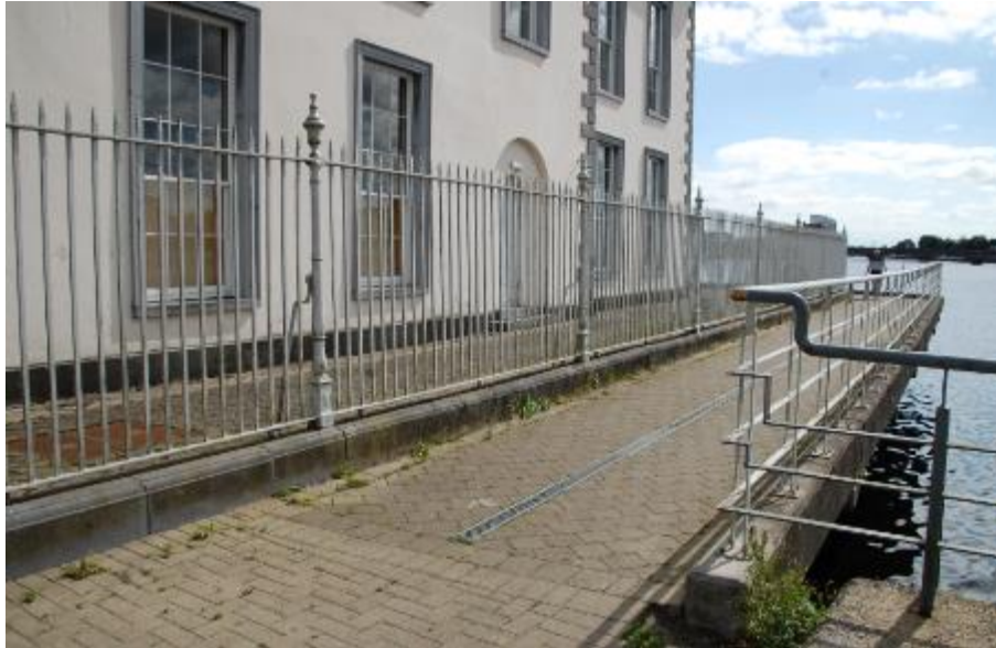
Plate 14-58. View of the north-eastern side of the County Court House, with replacement railings on original stone plinth and with modern boardwalk over the original quay wall
