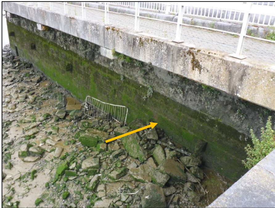
Photograph 4.1. Example of algal zone on quay wall (orange arrow)
