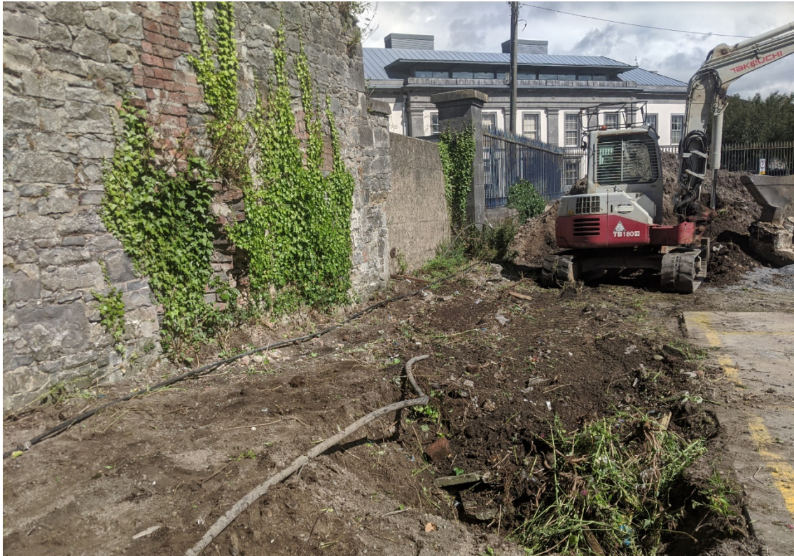
Figure 51 Location of TT4-1, facing north, with rear wall of Curragower Boat club to left.
