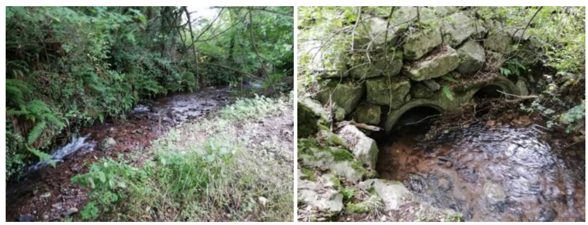
Figure 5-3. Cúil Chluthair culvert location (Left: looking upstream, right: looking downstream at existing culvert)
