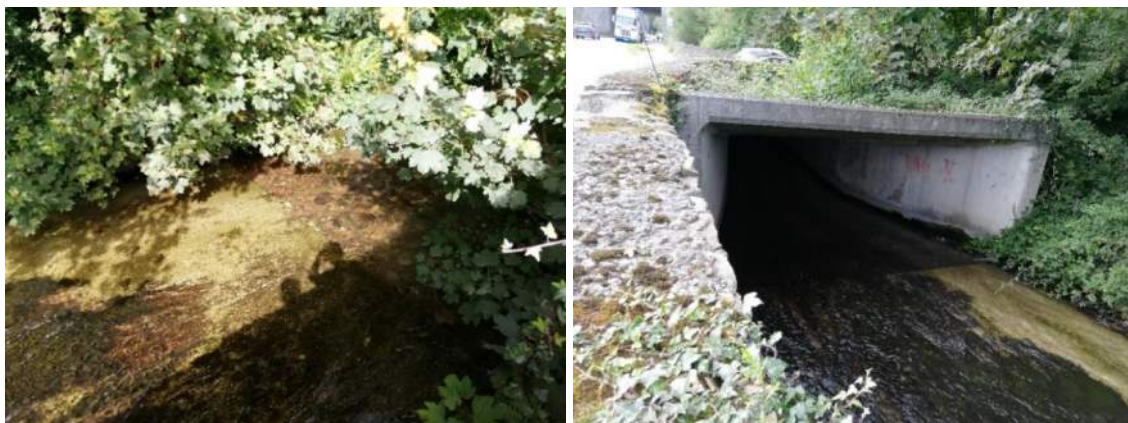
Figure 5-21. High gradient of culvert has resulted in bed scour at inlet of structure
