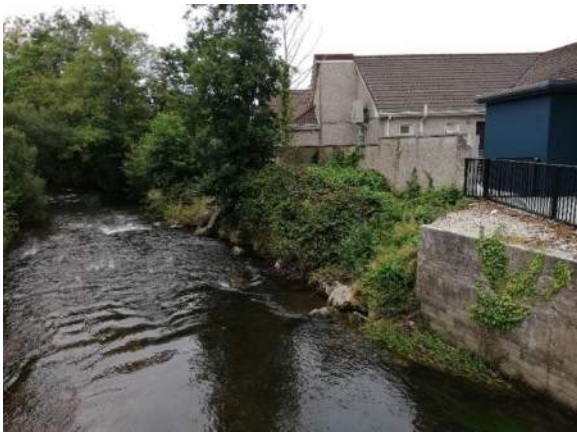
Figure 5-8. Existing retaining wall and rock armour to be replaced by RC walls (looking downstream at right bank)
