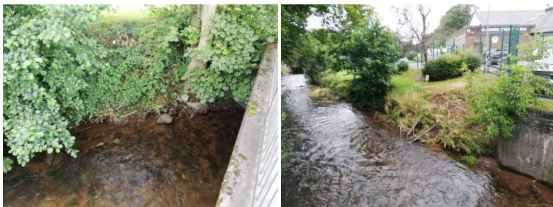
Figure 5-10. Bank instability noted around existing Hazelwood shopping centre bridge at downstream (left) and upstream (right)
