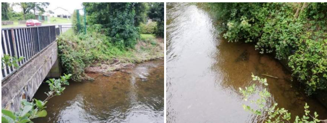
Figure 5-7. Location where new flood relief culvert to tie into existing bridge (left: bank failures observed at downstream,
