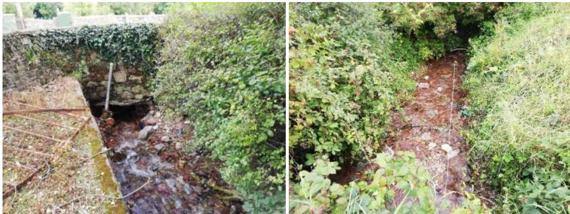
Figure 5-6. Existing culvert system at Cois na Gleann (Left: upstream end of culvert, right: downstream reach)
