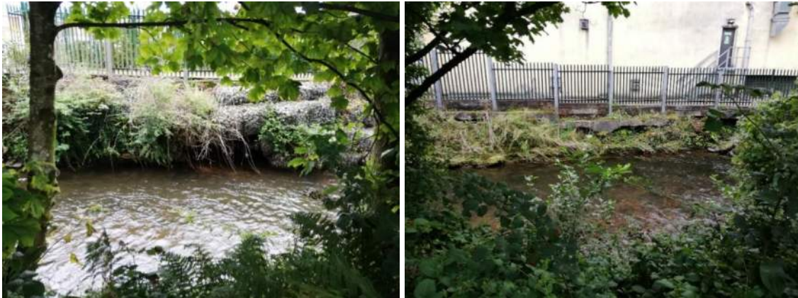
Figure 5-11. Undermining of ad-hoc defence structures observed on left bank
