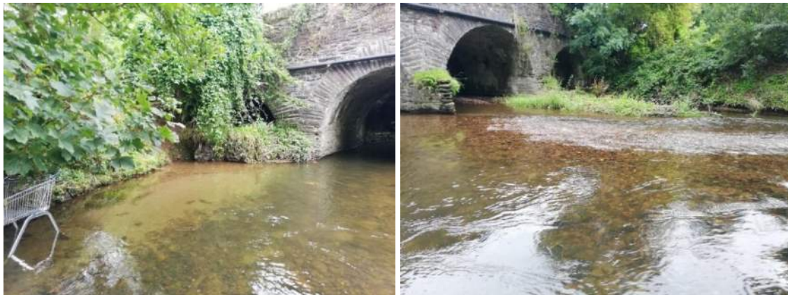
Figure 5-14. Deposition at Riverstown Bridge is primarily mid-channel gravel bars, with some fine sediments downstream of the east bank arch where outfalls are located and backwatering likely occurs during higher flows
