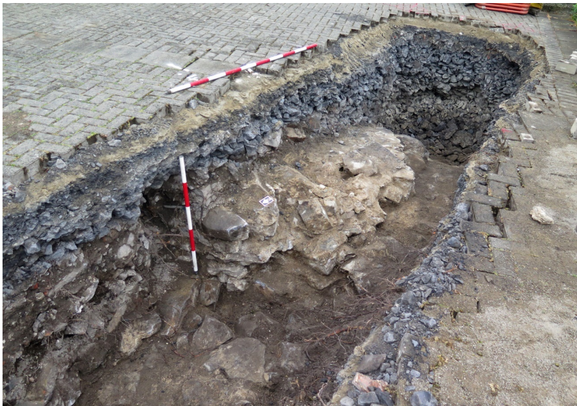
Figure 35 Looking south to bridge rubble core, not clean stone fill from 1980's infill.
