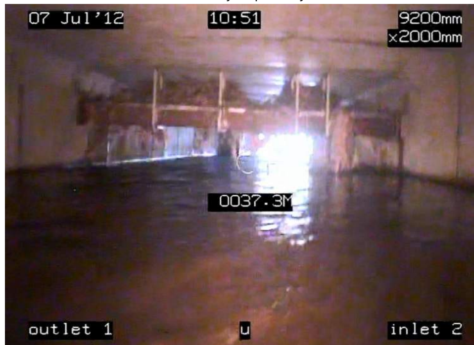
Photograph of ESB services tray in Orchard Court Culvert
