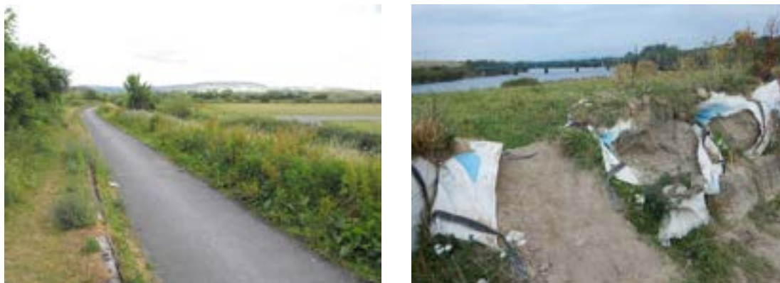
Figure 5-6: Existing flood embankment with damaged sandbags
