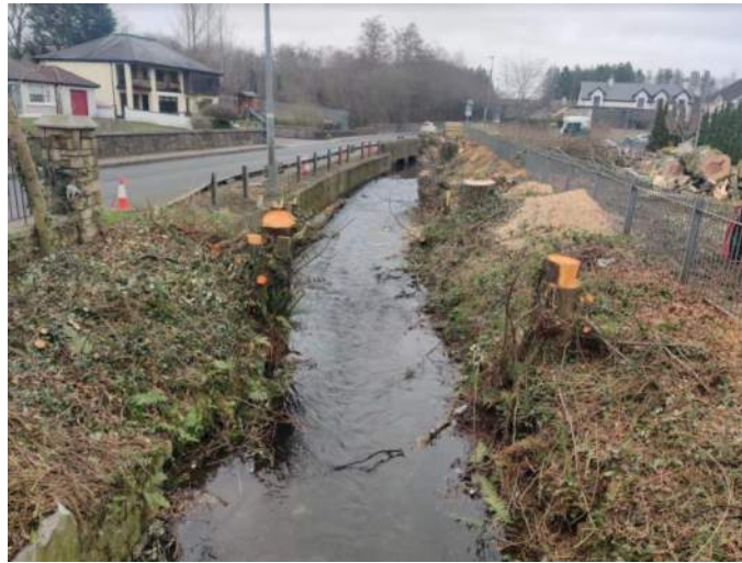
Site tree-felling and localised mulching and briar clearance. Felling completed and tree base and roots left in situ.
