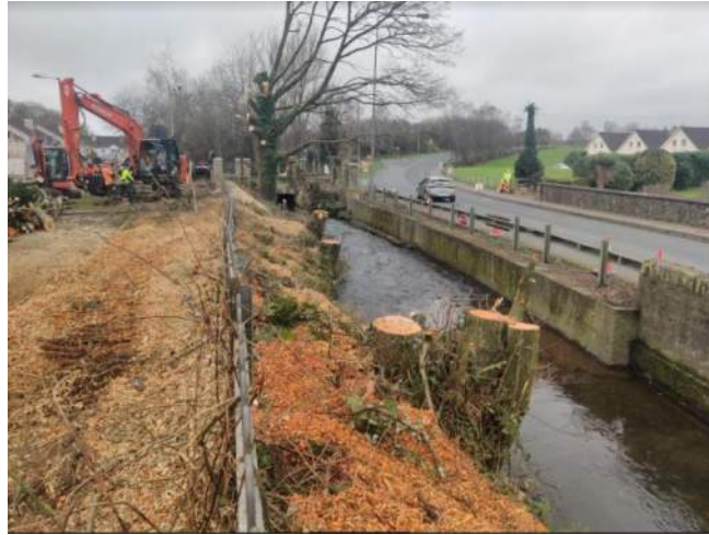
Site tree-felling and localised mulching. Felling completed and tree base and roots left in situ.
