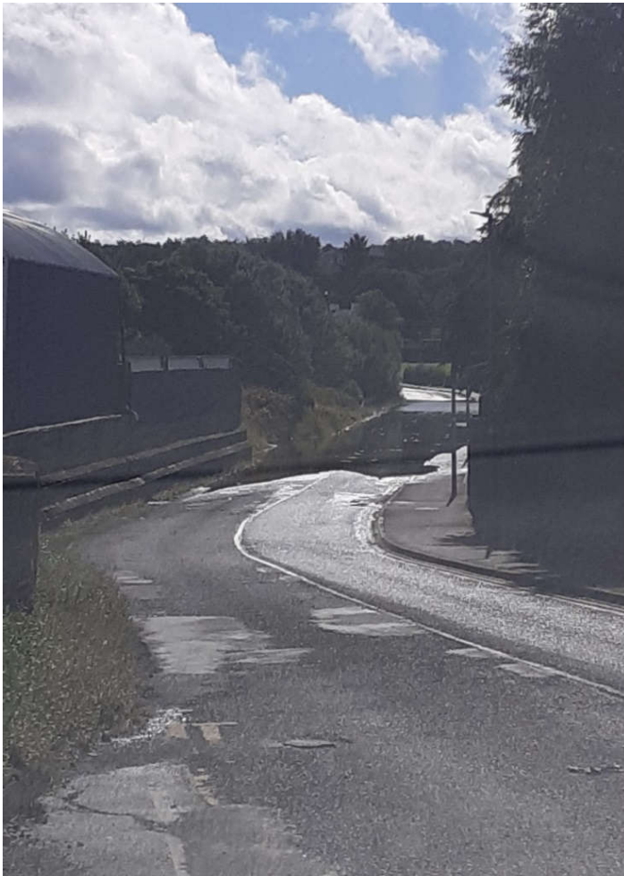
Minor Flooding on Navenny Street/Road, Ballybofey-Stranorlar – September 2022.
