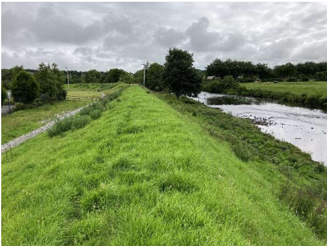
A recent photograph of the current condition of a section of the embankment near Finn Park, Ballybofey (June 2022)
