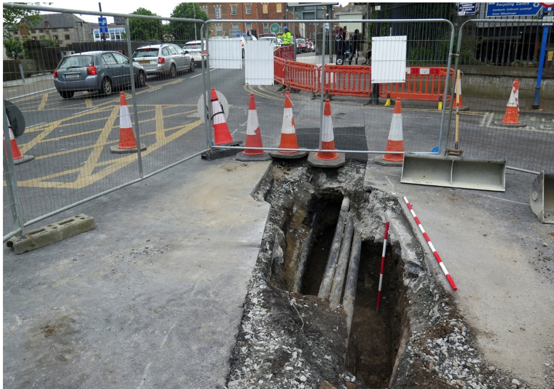
Figure 117 TT6-1 B Looking towards Potato Market showing ducts and foundation at base of trench, fresh tar at centre of carriageway shows extent of TT6-1 A
