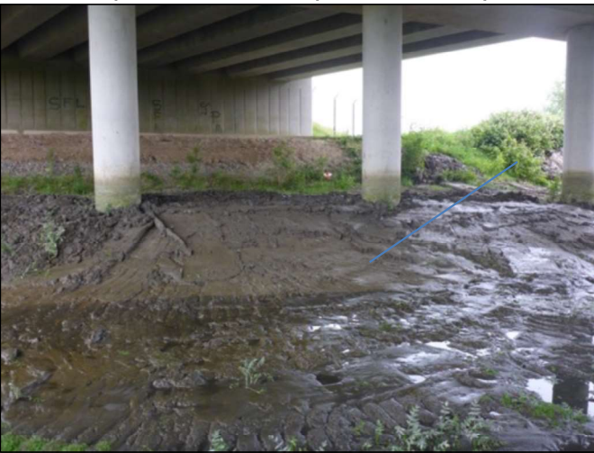
Photograph 1.15. Recent dredging/ disturbance under N18 bridge (view E from W bank)
