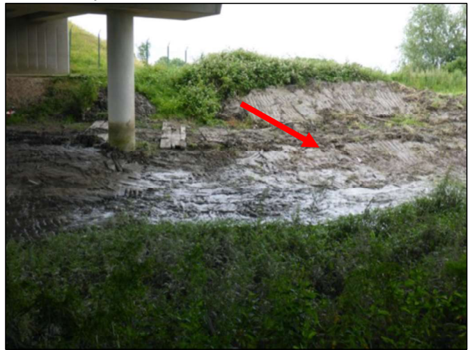
Photograph 1.16. Recent dredging/ disturbance to south of N18 bridge (red arrow, view SE from W bank)
