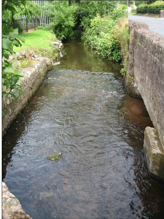
Plate 5: Glenmore Stream eastern section with garden to north (left) and Brooklodge Grove Road to south (right). Opening to the rectangular culverted channels are visible at bottom right, looking east
