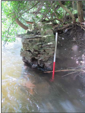
Plate 140: Southwest-facing view of eroded northern terminus of Feature F04B (1m scale).
