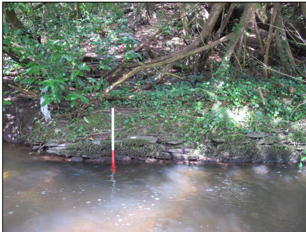
Plate 137: Eroded remains of a 4.9m section river-walling (Feature F04A) located immediately downstream of Feature F04B (1m scale); see Figure 11 for location.
