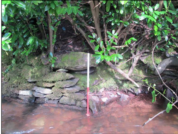
Plate 136: Eroded section of river-walling (Feature F04A) located short distance upstream of Feature F05 (1m scale).
